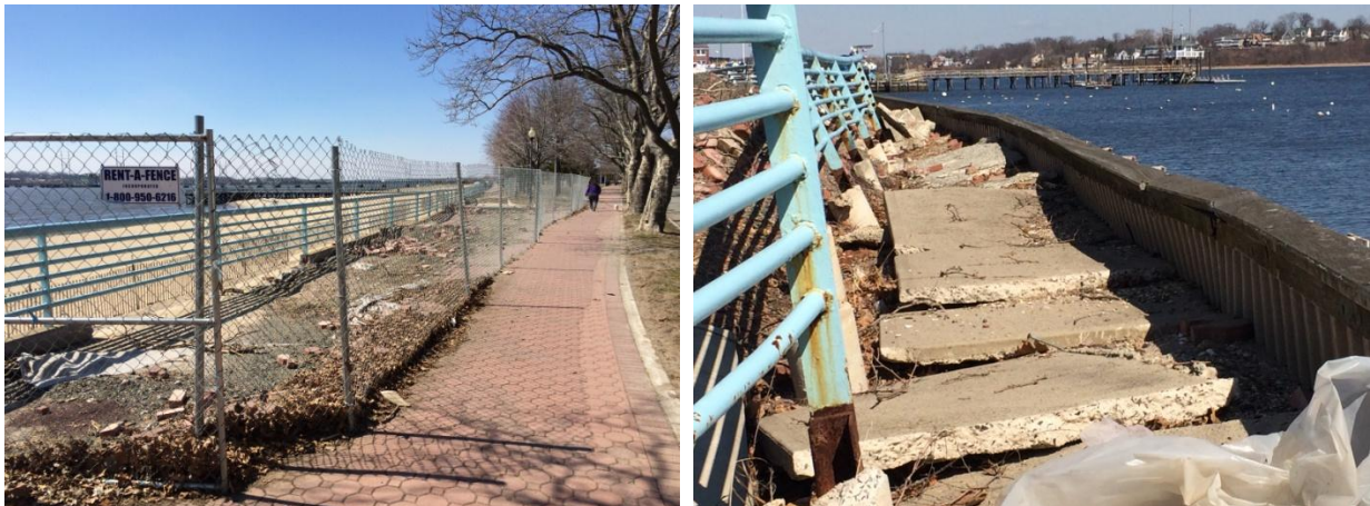
Figure 3: Much of the storm damage to public property was to sidewalks, bulkheads and railings along Perth Amboy's waterfront parks. The views above were taken in February of 2014 and show that recovery is still in progress and much remains to be reconstructed.
